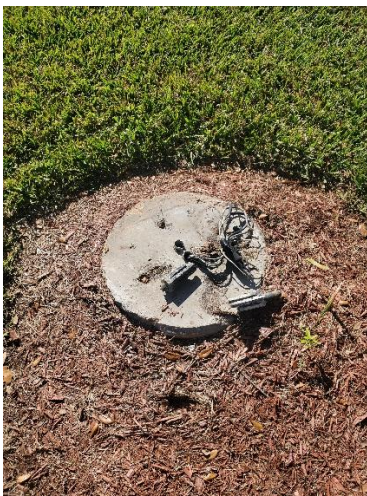
1.10.23 Pole 11 Foundation damaged
