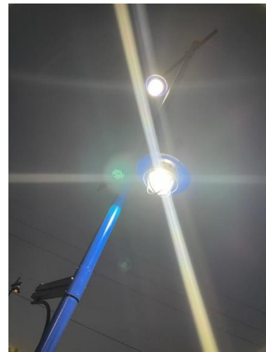
1.10.23 Pole #29 Pedestrian light operating
