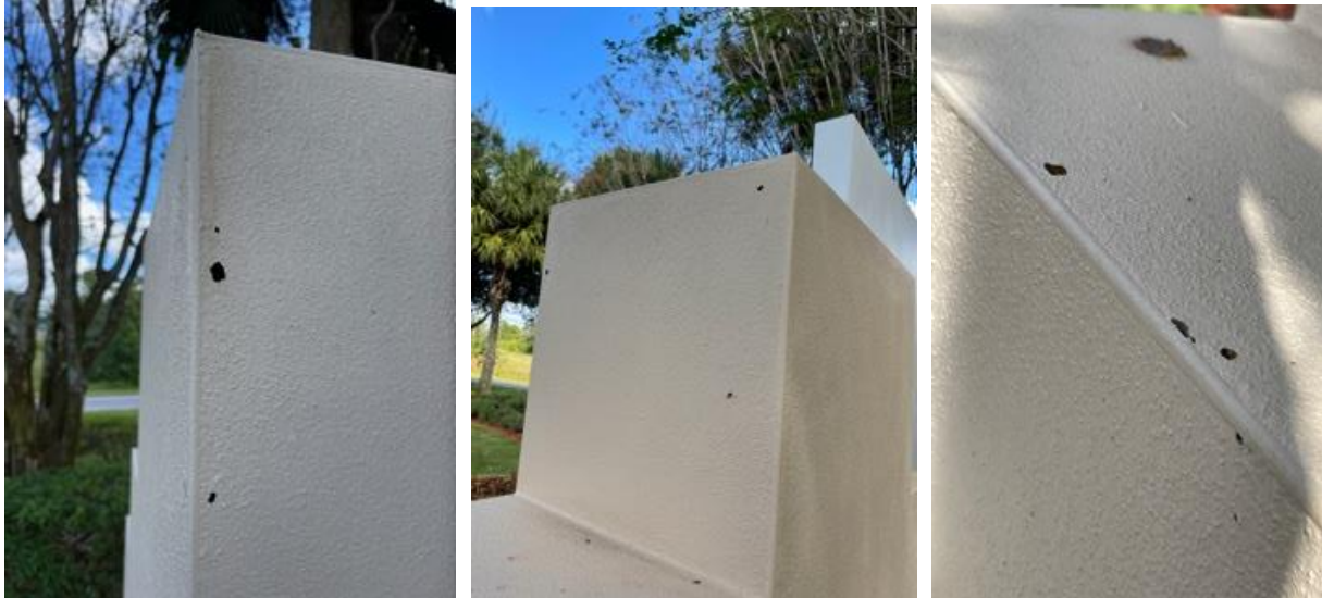
Stucco Failure at Triangle Monument 11.16.21
