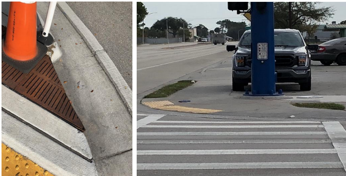
1.10.22 grates and ADA Pads in need of replacements
