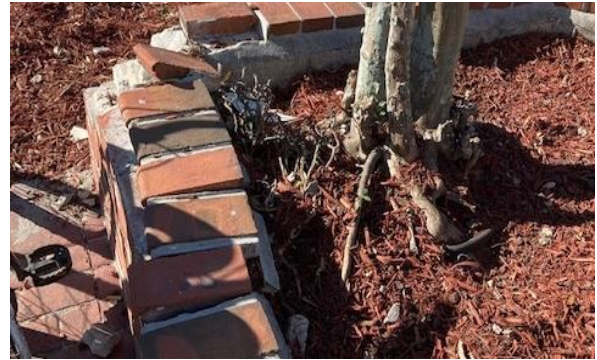
02.13.23 damaged bulb out planters
