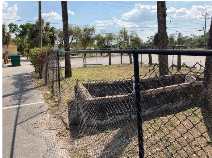
03.06.23 Fence damaged. May required professional services for repair
