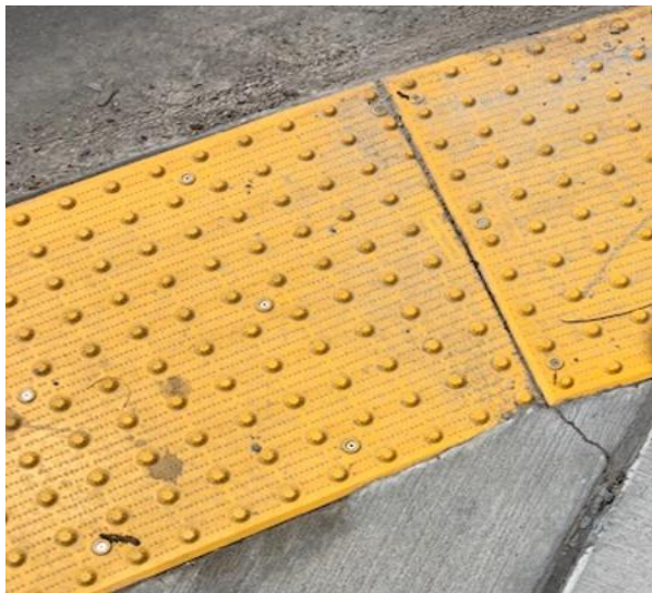
03.17.22 crack under ADA mat NE corner of Eustis/S 5 th
