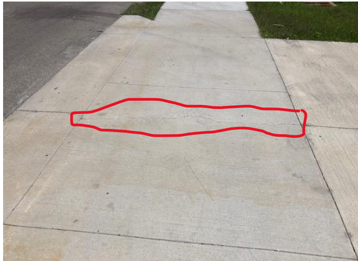
03.17.22 cracked sidewalk on South side of Carver (Guadalupe property)
