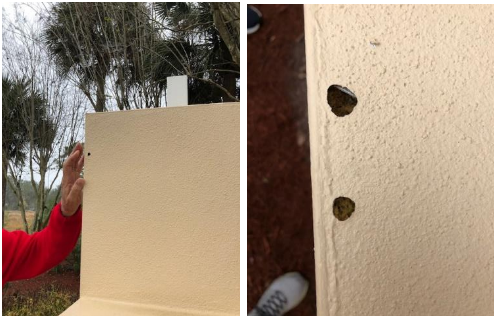
02.07.22 perimeter holes on monument sign
