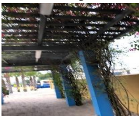
Trellis 3 florescent lights
