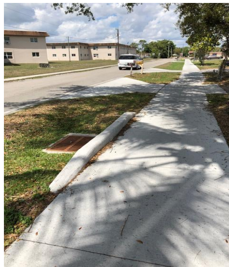
03.17.22 S 5 th St requires a handrail on stem wall
