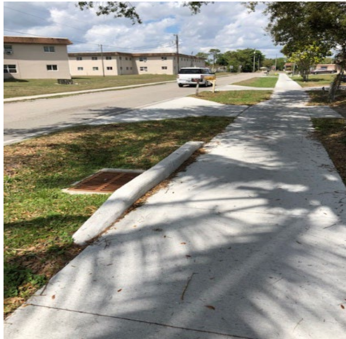
03.17.22 S 5 th St - Post Final Completion a handrail and footer are recommended
