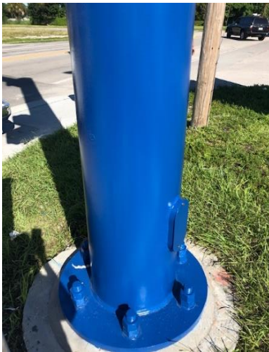
10.13.21 NE signal pole Main/9 th
