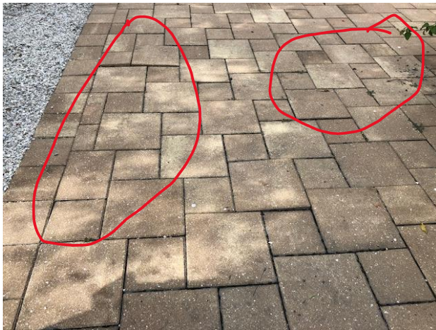
Uneven pavers identified on June 7, 2021
