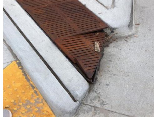
Damaged Grate at Curb Main-2 nd St S. 6.2.21
