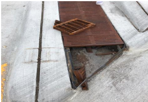
Damaged Grate at Curb Main-4 th St S. 6.2.21
