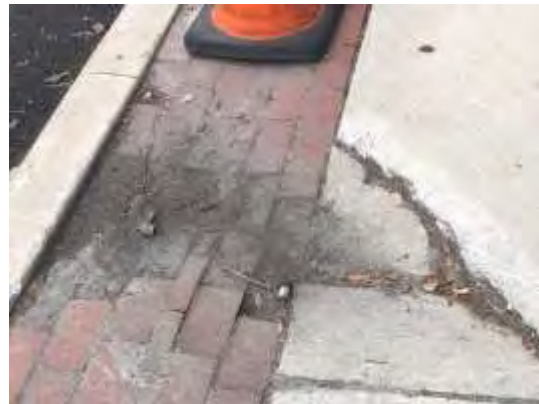
10.18.22 Sunoco sidewalk to be replaced
