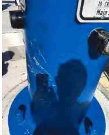
09.16.22 damaged mast arm pole
