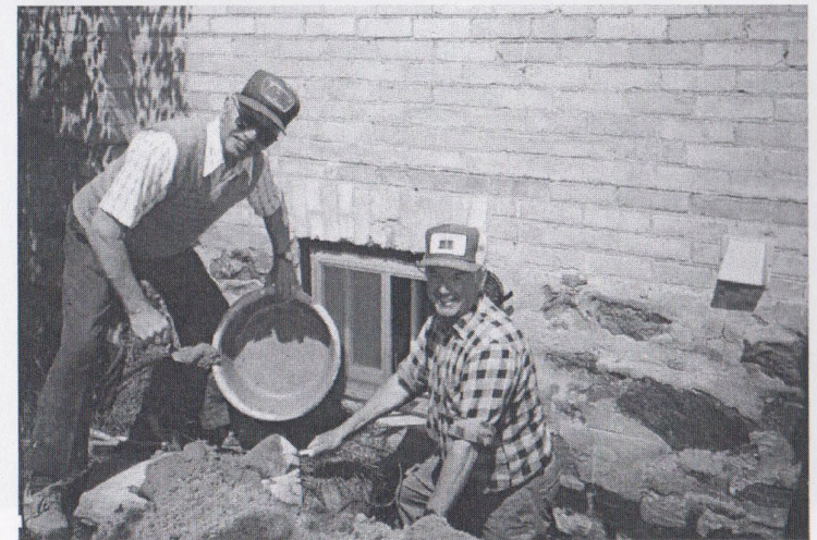
Henry Fleischbauer (left) and Don Rutz repairing the foundation of the Lutheran Student House, 1995
