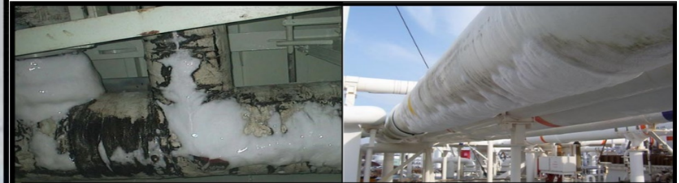
Water in insulation layers becomes ice and crushes Insulation cell material Locations where water accumulates in insulation layers will crush insulation cells and create worse and worse situation for each cool down.
