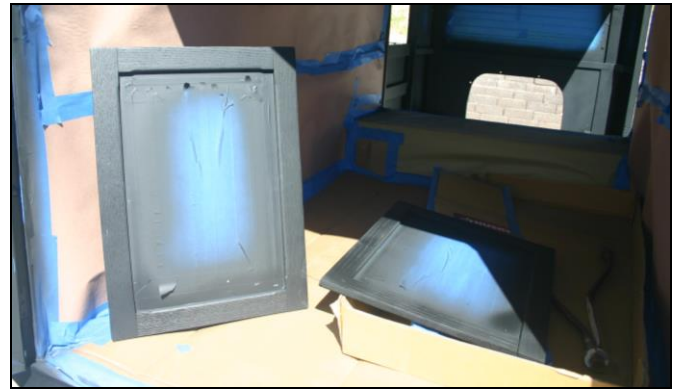
Tom masked off the glass of the cabins' lift windows, sanded and filled the wooden frames and applied their first prime coat.
