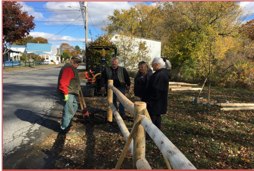
Charlie Poulin stopped by to help WCLT install the new fence. (Left to right: Charlie, contractor Doug Kane and his assistant Sam, and WCLT President Paula Saul. Picture by Nancy Williams.)
