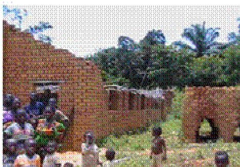
Church being rebuilt using locally made and fired bricks. On the right is a kiln made of the mud bricks to be fired.
