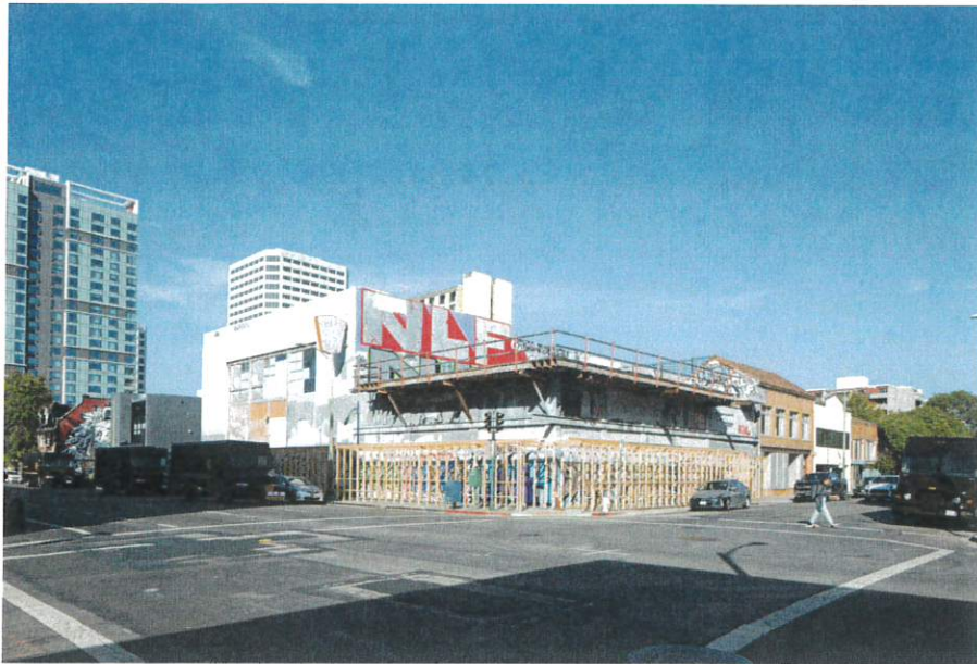
1510 Webster Street site prepares for demolition with the protective shed now rising, image by author
