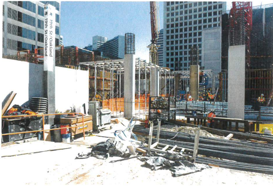
1900 Broadway construction site with the existing 19th Street BART Station remaining active throughout the project, image by author
