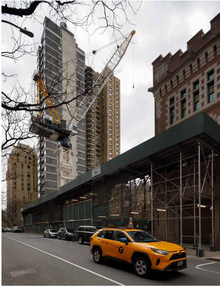
The construction site at 50 West 66th Street, where a planned 775-foot tower is being held up by challenges from community groups that argue the developer will build excessively tall mechanical rooms to add height — nearly 200 additional feet — to create a premium for its priciest condo units on higher floors. Stefano Ukmar for The New York Times
