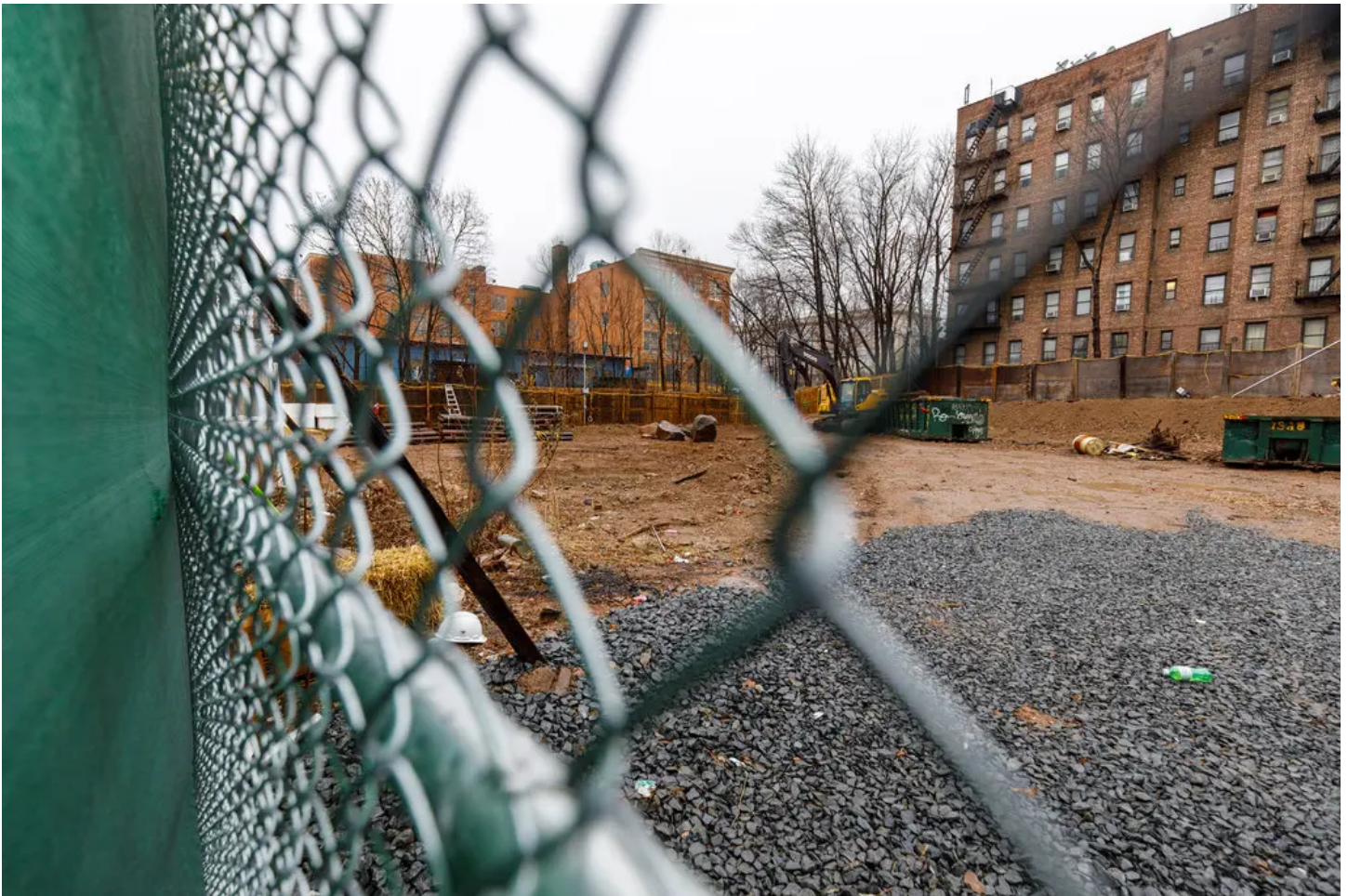
The construction site at 931 Carroll Street in Crown Heights, where a judge decided to temporarily halt construction until a more thorough review of the plans could be conducted. Stefano Ukmar for The New York Times
