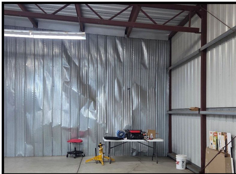
Hangar Interior Wall Buckling
