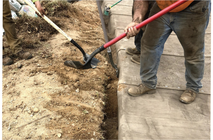
The team digs a trench to help anchor the Concrete Cloth GCCM into the ground
