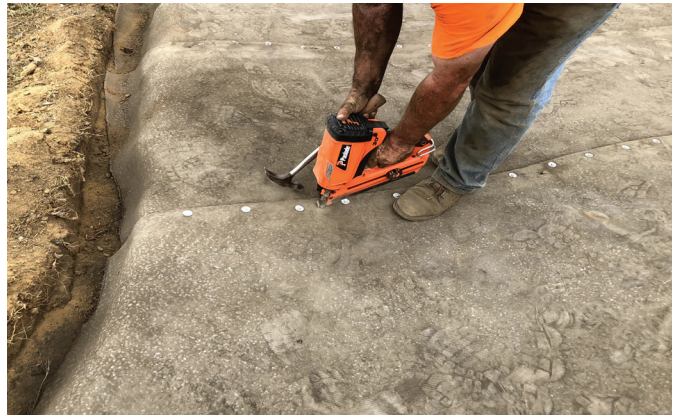
The material is anchored to the existing asphalt channel using four-inch nails
