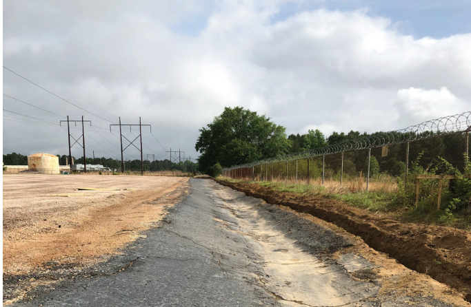
Asphalt swale before rehabilitation
