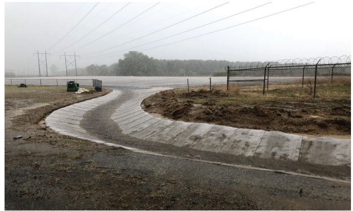
The contractor used the weather conditions to his advantage to hydrate the Concrete Cloth GCCM because it cannot be over-hydrated
