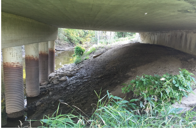
Initial slope conditions with erosion near columns.
