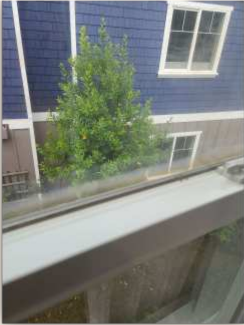
A failed energy cutting noted at the second floor window on the west side.
