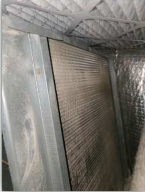
This shows an evaporator coil that was likely never used
