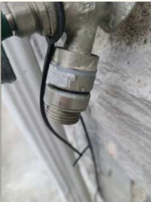
This shows the anti-siphon present at the garage side hose bib
