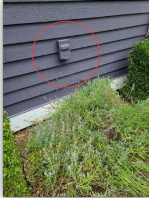
This appears to be an electrical disconnect that may have been designed for a heat pump
