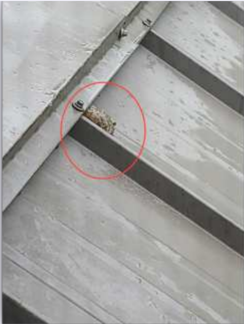
This was at the south side ridge
