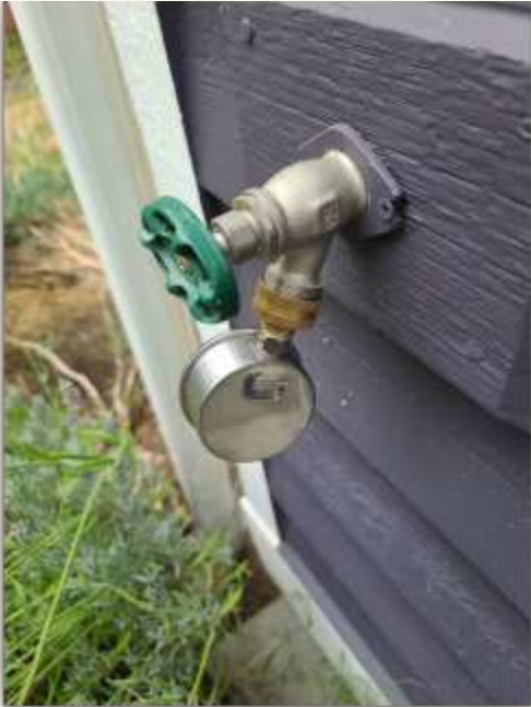
The anti-siphon device is missing for the backyard hose bib.
