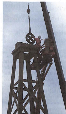
Crown pulley installed
