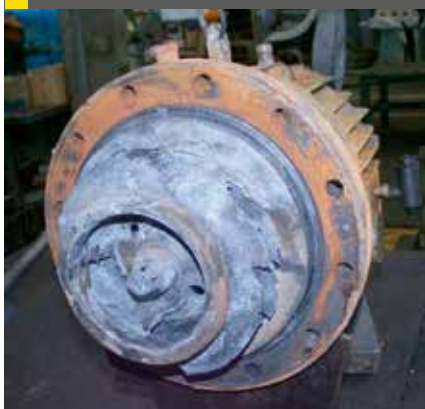
Fig 7: Reflux pump corrosion due to elevated salt content
