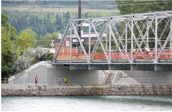
The Shouldice Bridge in Bowness. At the time of the June 20 flood, the raging Bow River nearly touched the bottom of the bridge's surface. Michelle Hofer / For Inner-city Living
