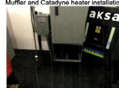
Wiring of Transfer Switch
