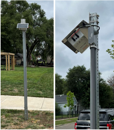
Data Acquisition Computer, Battery, Solar Panel & Stand-Alone Pole
