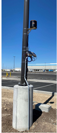
Existing Pole Mounting
