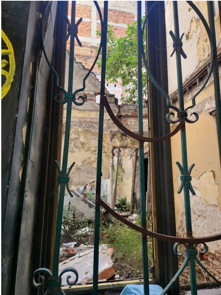
Abandoned structure in a central area in the Roma/Condesa area. Photos by Ernesto Castañeda. November 15, 2024.
