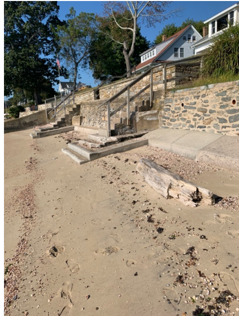
11 Chapman Ave. Surmolian
