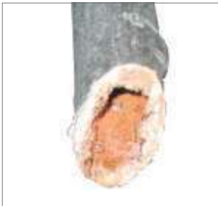
Corrosion build-up in metal pipes
