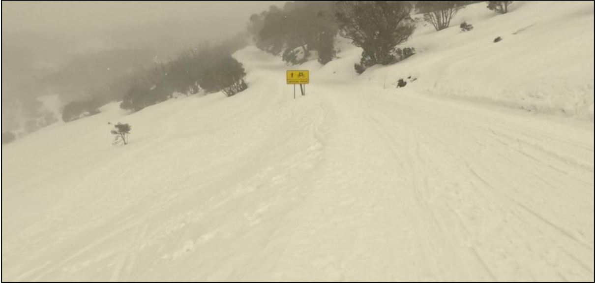
The section of road that has slipped
