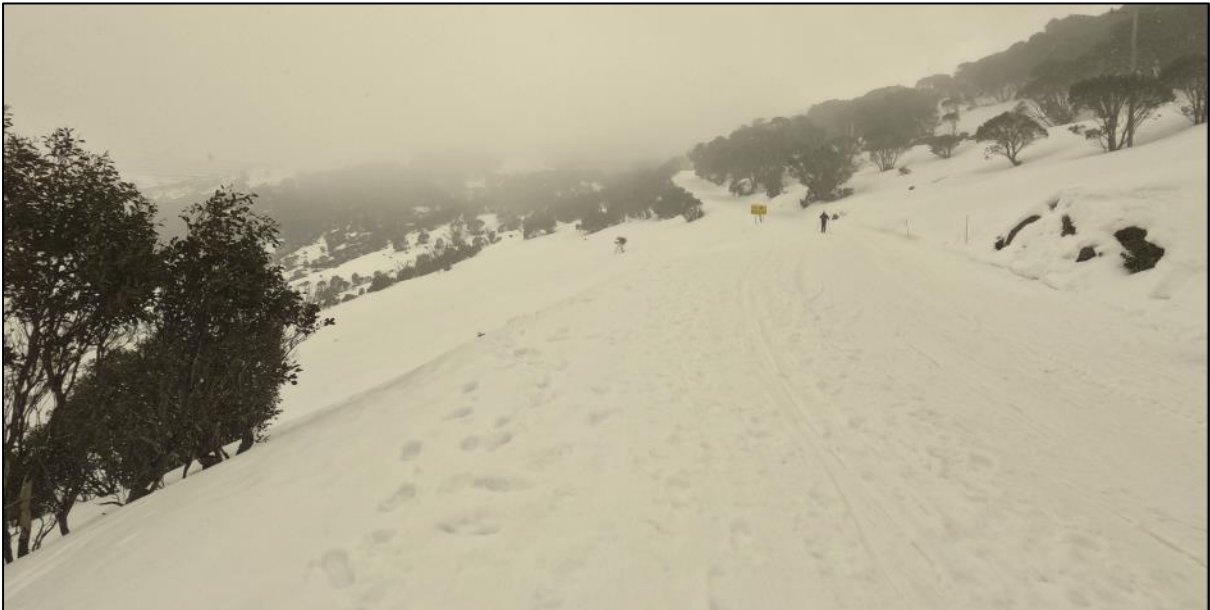
Towards the area of the road that has slipped
