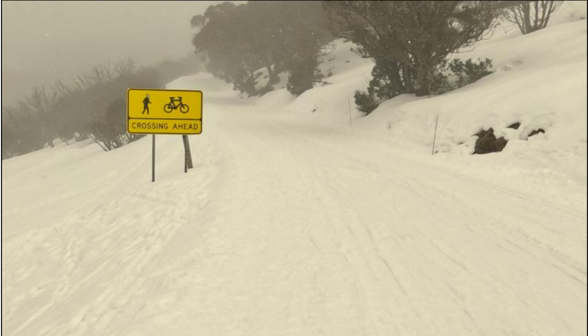
The section of road that has slipped
