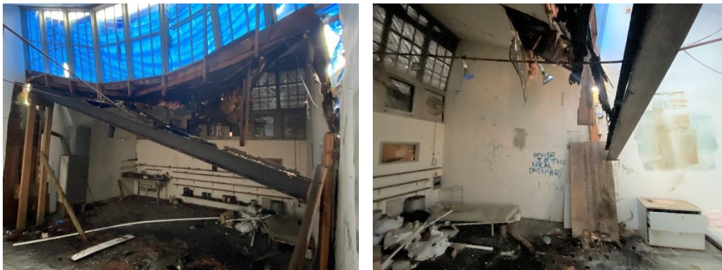
Photo No. 18 and 19: Chronic water infiltration has resulted in significant damage to the roof and skylight.
