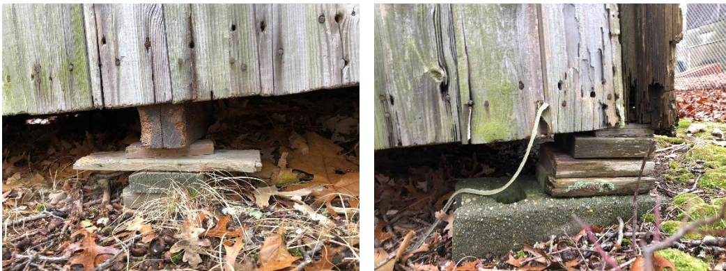
Photo No. 30 and 31: The foundation elements do not properly support the structure.
