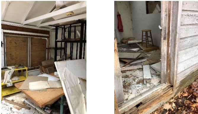
Photo No. 24 and 25: The window sash and frames are salvageable but will require re-glazing. The entry door is heavily damaged and will require full restoration.
