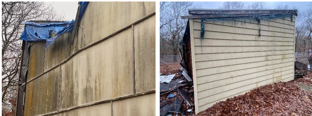
Photo No. 16 and 17: Note the distressed Transite panels where the "I" beam has failed. The aluminum siding is in good overall condition with only minor damage.
