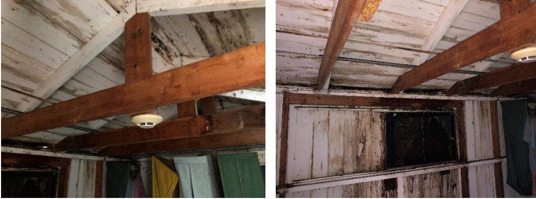
Photo No. 32 and 33: The ceiling and wall cladding is water damaged, but only requires preparation and repainting.
