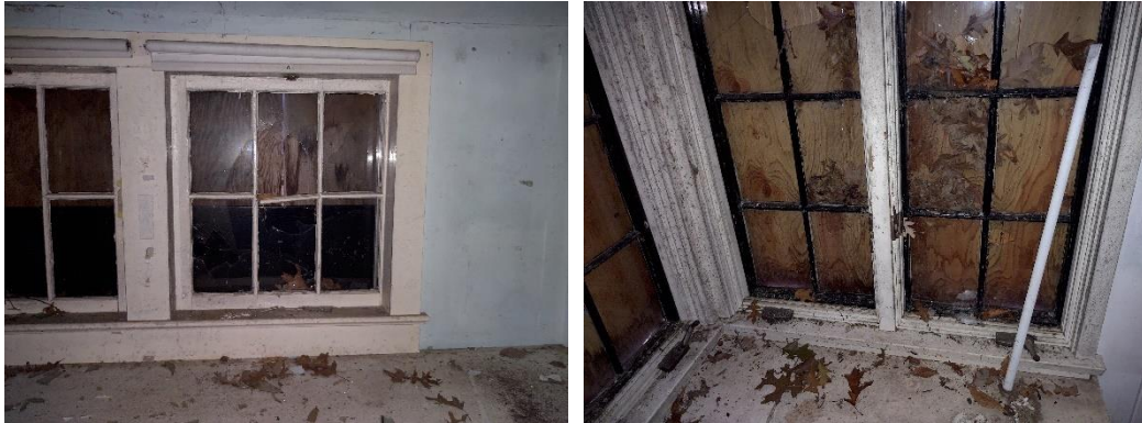
Photo No. 6 and 7: The windows all require some level of repair. While most only require re-glazing, some have damaged mullions requiring sash restoration.
