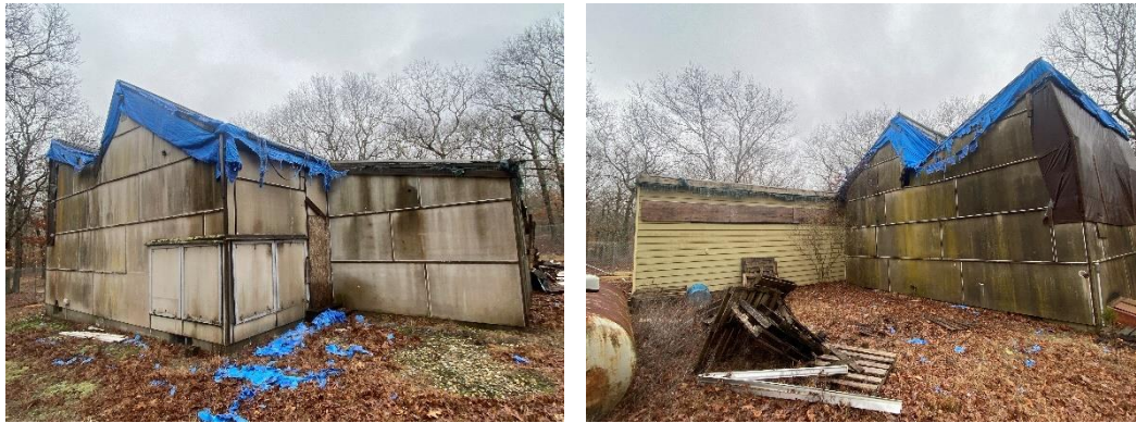
Photo No. 14 and 15: The Brooks Studio was built over two campaigns, the main block clad in Transite panels, and the SE storage wing clad in aluminum siding.
