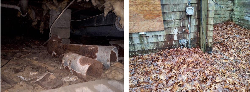
Photo No. 12 and 13: The building systems are non-operational and will require upgrades for any proposed re-use of the residence.
