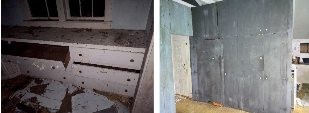
Photo No. 10 and 11: The cabinetry primarily requires only minor repairs and repainting.
