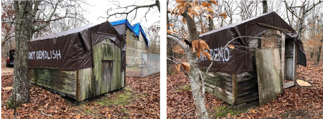
Photo No. 28 and 29: The guest cottage is a small wood framed structure located to the north of the Brook Studio.
