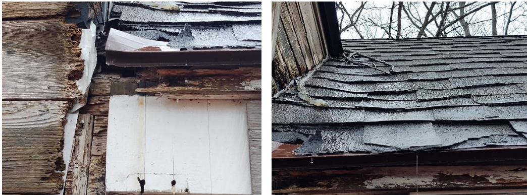
Photo No. 2 and 3: Asphaltic shingles have been installed over the original wood shingle roofing. There is extensive damage to the ceiling below this location.
