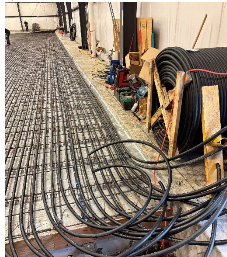
Brine lines at Home end to be connected to supply/return header
