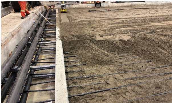
Brine supply/return headers on left. 10” of sand burying glycol lines.
