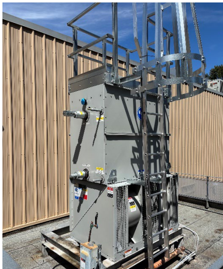
South side of new Evap Cond
