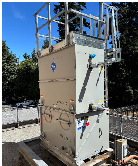
North side of new Evap Cond
