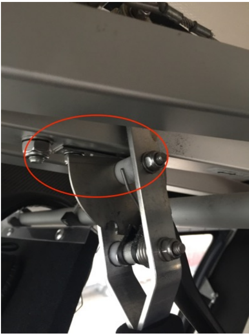
Photo 1: Crack from left hand side
