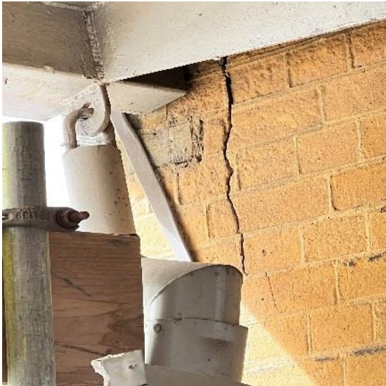
Existing masonry interface identified for repair
