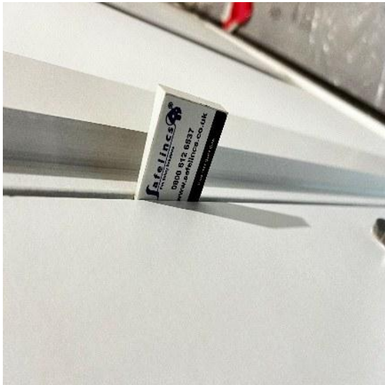
Fire door certification label and installation evidence
