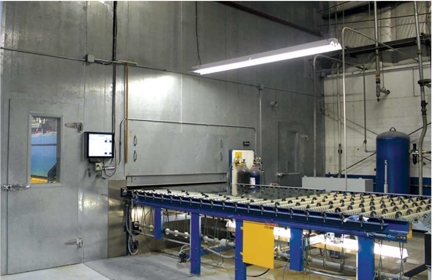
Rollers feed the glass into the tempering oven. Also referred to as "safety glass," tempered glass, shatters into small cubes when broken, as opposed to jagged shards.
