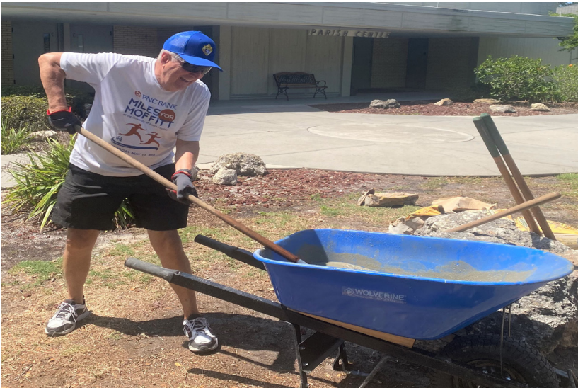
Bill Bannon takes his turn to mixing cement. All the Knights were worn out after a long day of hard work.
