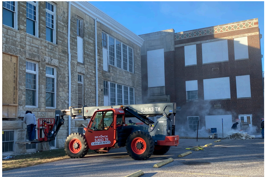
In the foreground, a construction crew member is carefully fitting a limestone block into the opening above the window. In the background to the right, another crew member is shaping a limestone block with a stone saw. Photo: Cynthia Rhodes
