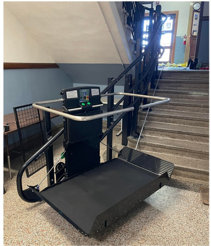
The newly installed Garaventa Artira inclined platform lift. Photo: Paul Oberg
