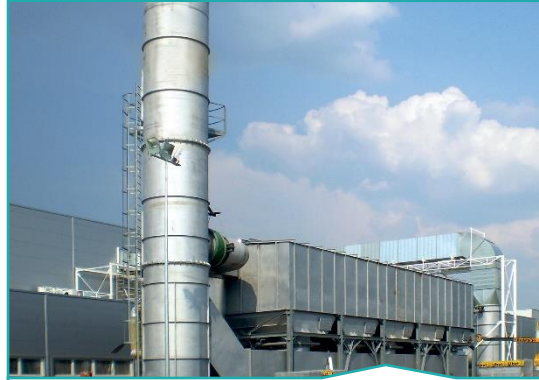
S2 – Vapor Combustion Unit
