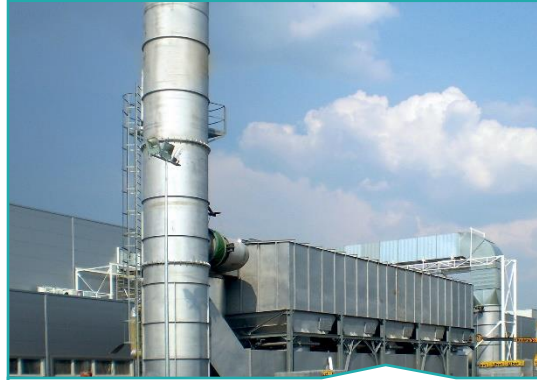
B2 - Vapor Combustion Unit
