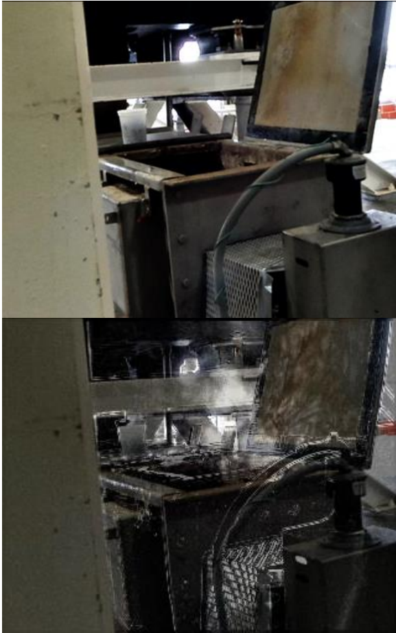
Dewatering Centrate Chute
