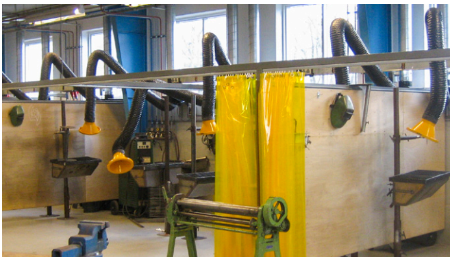
Wing arms ø160mm 3m installed at technical school. Including automatic control devices for automatic start/stop of fan and motor damper.
