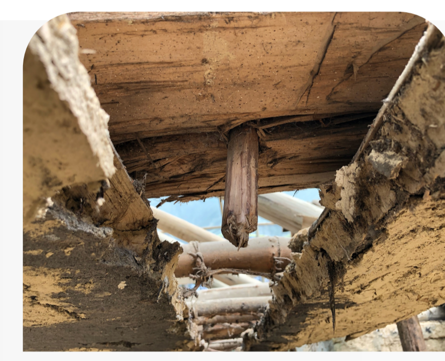
Both houses featured the doweling technique, which uses wooden joints such as tenons and mortises to fit pieces together.
