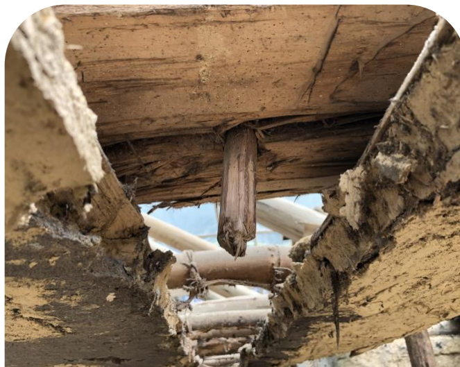
Both houses featured the doweling technique, which uses wooden joints such as tenons and mortises to fit pieces together.
