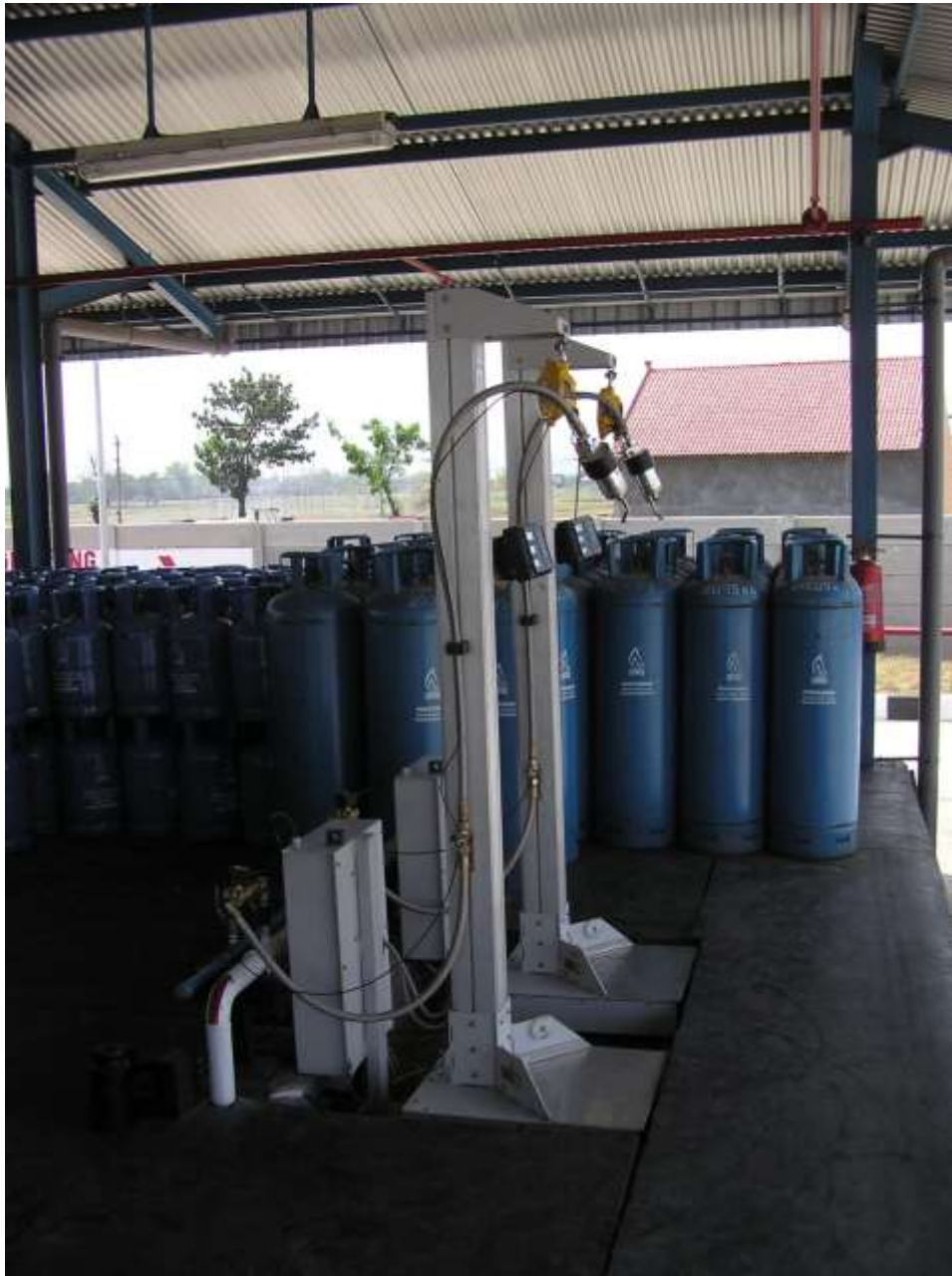
ELIXIR Stationary Filling Machines for 50-kg cylinders installed in Indonesia
