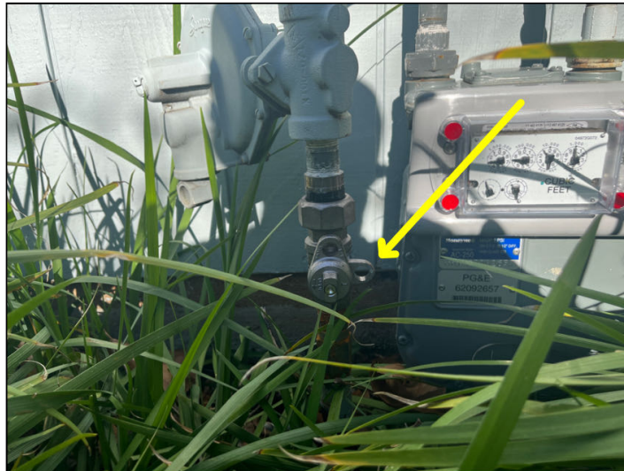
This is the gas shut off valve located on the meter itself.
