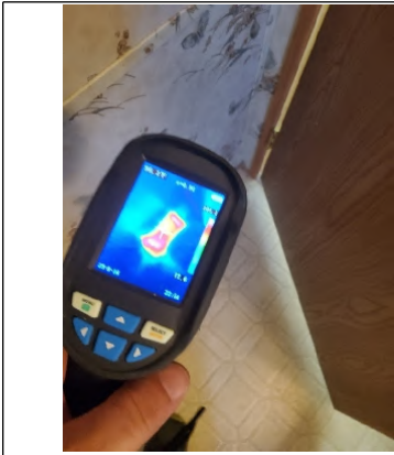
Thermal Imager shows proper "Heat" distribution through vent along with properly sealed ducting at the register.
