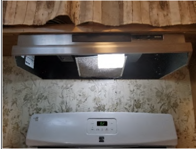
Exhaust fan is noisy and should be repaired by an Appliance Specialist.
