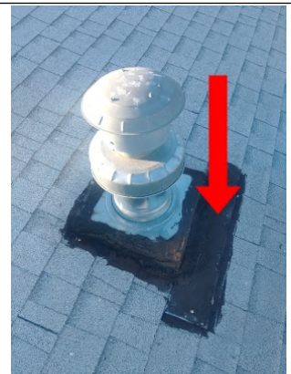
Henry's roof sealant was applied for flashing. This would have to be reapplied every 3-years I would recommend resealing it with a much better product like Black Jack Rubr-Coat.
