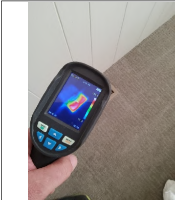
Thermal Imager shows proper "Heat" distribution through vent along with properly sealed ducting at the register.
