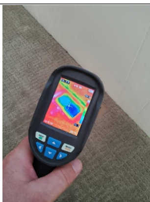
Thermal Imager shows proper "Cool" distribution through vent along with properly sealed ducting at the register.
