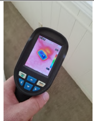
Thermal Imager shows proper "Cool" distribution through vent along with properly sealed ducting at the register.
