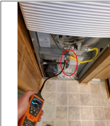
No leaks were detected at shut off valve.
