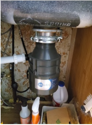
Garbage disposal shows proper operation
