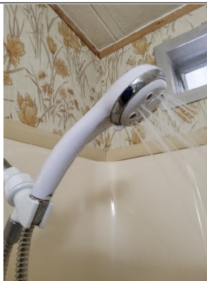
Shower head has a leak. Recommend having repaired or replaced by a Licensed Plumber.
