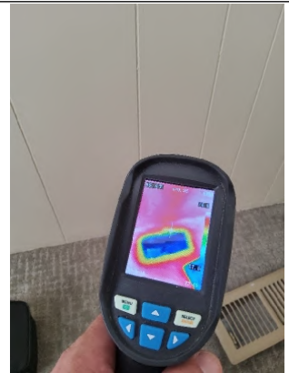
Thermal Imager shows proper "Cool" distribution through vent along with properly sealed ducting at the register.
