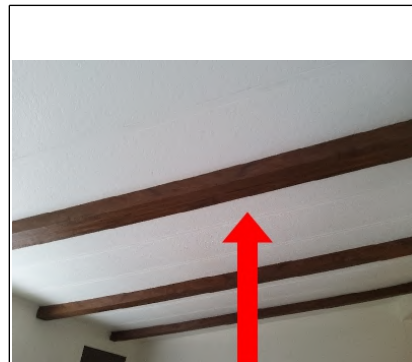
Dips in the ceiling are cosmetic these beams are not structural as there are spanning joist members above them that meet at the ridge point.
