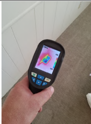
Thermal Imager shows proper "Cool" distribution through vent along with properly sealed ducting at the register.
