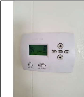
Thermostat shows proper operation on "Heat" setting.
