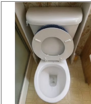
Toilet is loose at the base. Recommend properly fastening to the floor by a Licensed Plumber.
