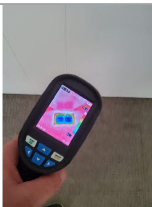
Thermal Imager shows proper "Cool" distribution through vent along with properly sealed ducting at the register.
