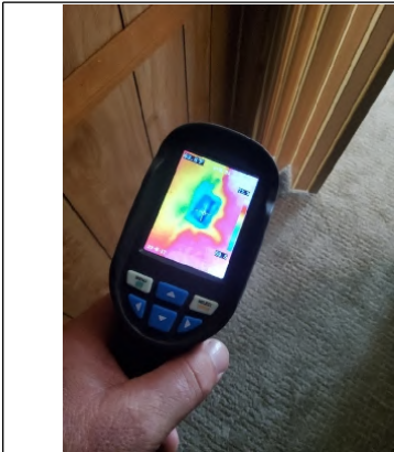
Thermal Imager shows proper "Cool" distribution through vent along with properly sealed ducting at the register.
