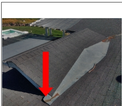
Recommend fastening this section of flashing on the valley in the roof sheathing washer head sheetmetal screws and a dab of sealant ontop of the heads.
