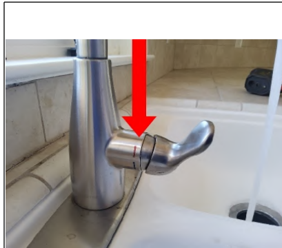
Hot and cold water lines are backwards. Recommend having a Licensed Plumber switch flex line water supply lines to correct locations.
