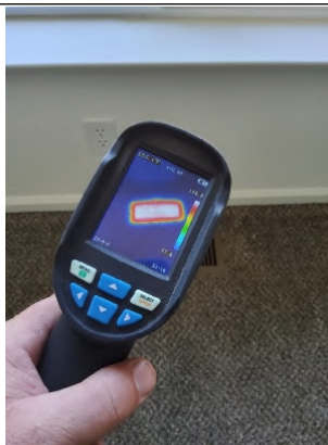
Thermal Imager shows proper "Heat" distribution through vent along with properly sealed ducting at the register.
