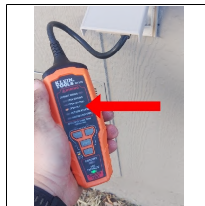
GFCI is inoperable. Recommend having replaced by a Licensed Electrician.
