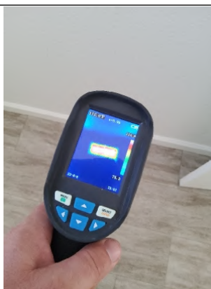
Thermal Imager shows proper "Heat" distribution through vent along with properly sealed ducting at the register.
