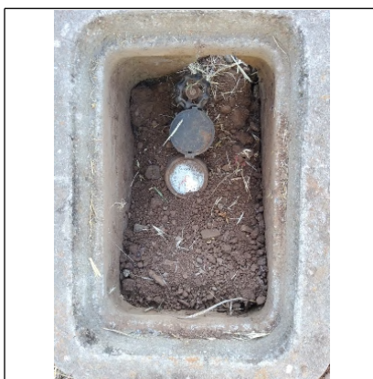
Recommend clearing dirt back to properly access shut off valve.
