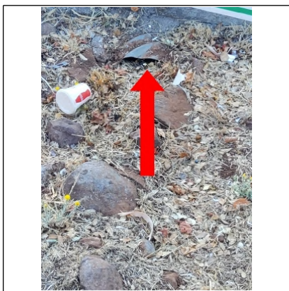
Recommend clearing dirt away from culvert drain.
