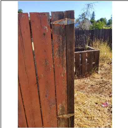
Recommend replacing gate hinges.
