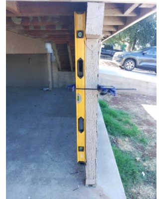
Column is slightly leaning but is of no structural concern.
