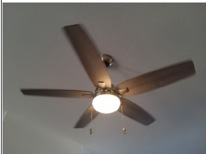
Ceiling fan shows proper operation.
