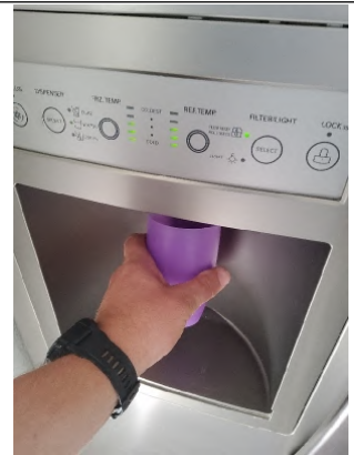
Water is currently not turned on for Ice Machine to properly operate or test.
