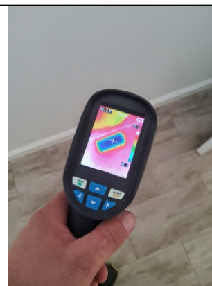
Thermal Imager shows proper "Cool" distribution through vent along with properly sealed ducting at the register.
