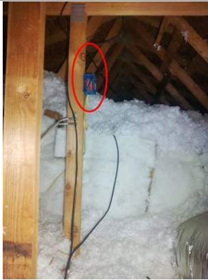
Recommend solid junction box be installed.
