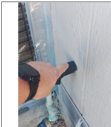
Copper line is slightly loose to siding. Recommend having properly fastened.
