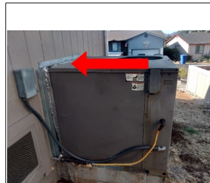
Recommend additional HVAC tape be applied
