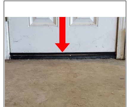
Recommend replacing existing door sweep with one that has a vinyl seal.
