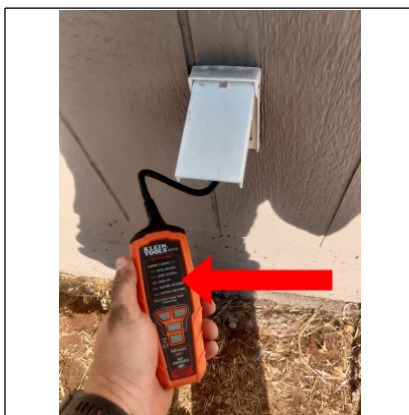
1. GFCI is inoperable. Recommend having replaced by a Licensed Electrician.
