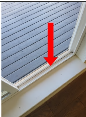
Recommend lubricating sliding door track with WD40 to ease the operation.
