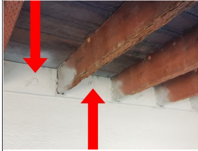
The deck is structurally sound. Galvanized 5/8" lags are placed every joist bay on the deck ledger to properly fasten to rim member of the home.
