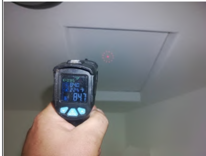
Thermal Reader shows 84.7 Degrees F on attic access lid.
