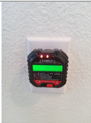
Electrical outlet shows proper operation, grounding and polarity.
