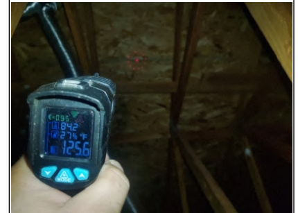
Thermal Reader shows 125.6 Degrees F at the OSB sheathing this shows there is proper ventilation and a moderate heat index.
