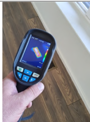
Thermal Imager shows proper "Heat" distribution through vent along with properly sealed ducting at the register.
