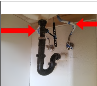
Recommend removing all painters tape from flex supply lines.
