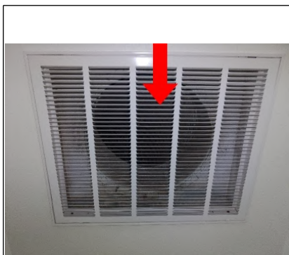
Missing cold air return filter
