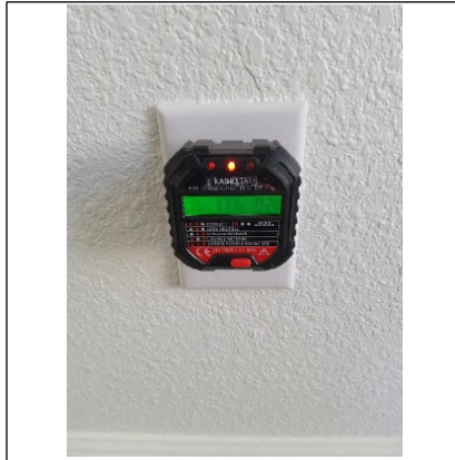
Electrical outlet shows proper operation, grounding and polarity.
