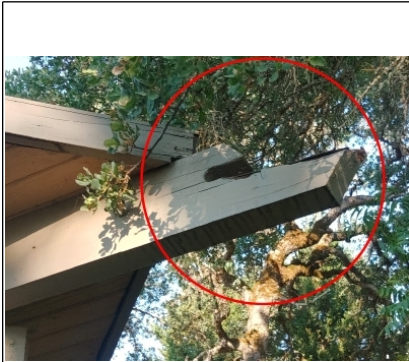
Recommend cutting back the moisture damaged exposed beam flush to fascia member.
