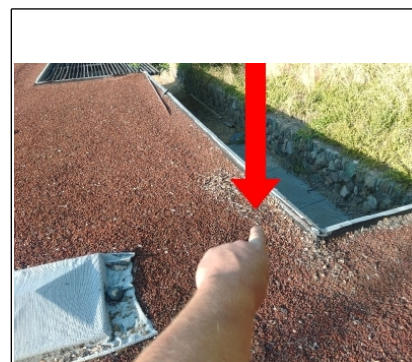
Recommend additional scupper drain and downspout location.
