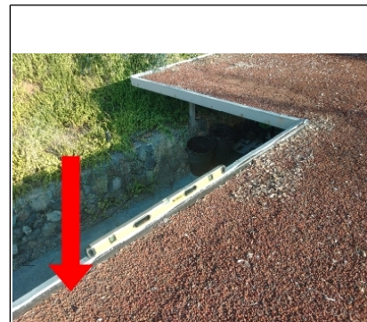
4' level is placed on the edge to show there is an improper pitch to the existing scupper drain.
