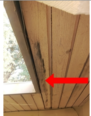
Moisture stains from active ponding location.
