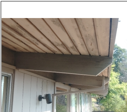
Significant bowing is evident on the T and G planking at the front portion of the overhang.
