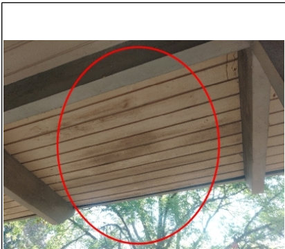
Significant bowing is evident on the T and G planking at the front portion of the overhang.
