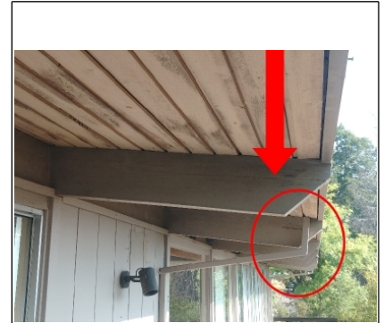
Moisture stains are evident on fascia from moisture intrusion through the tongue and groove planking.
