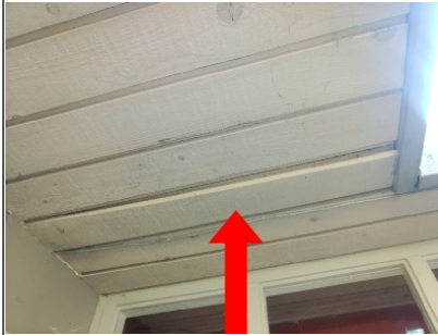
Disconnected planking member.
