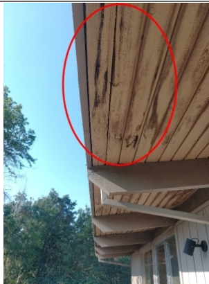
Stains are from water intrusion between the grooves of the planking.
