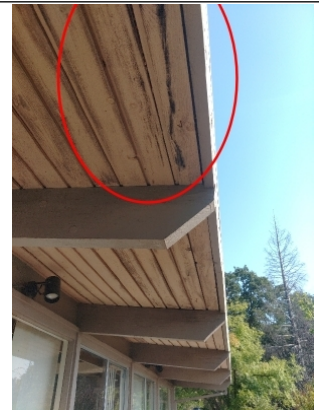
Stains are from water intrusion between the grooves of the planking.
