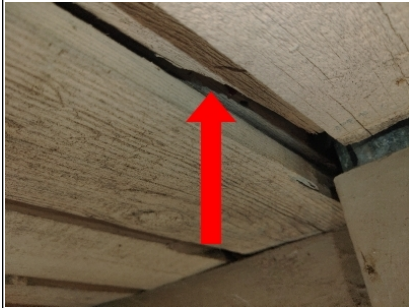
Another concern is that after this long winter and now this summer these exposed T and G planking members have shrunk. These are 1-1/2" wide T and G planks.
