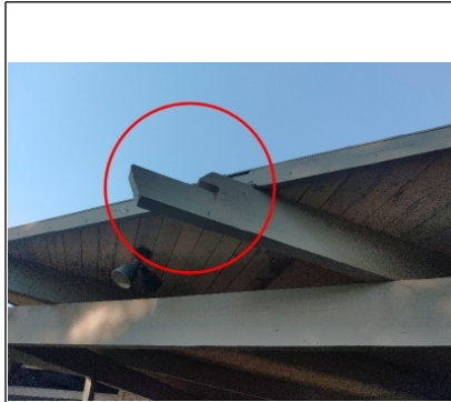
Recommend cutting back the moisture damaged exposed beam flush to fascia member.
