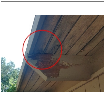
Moisture stains are evident on fascia from moisture intrusion through the tongue and groove planking.
