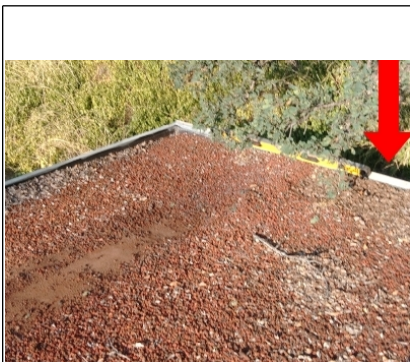
4' level is placed on the edge to show there is an improper pitch to the existing scupper drain.
