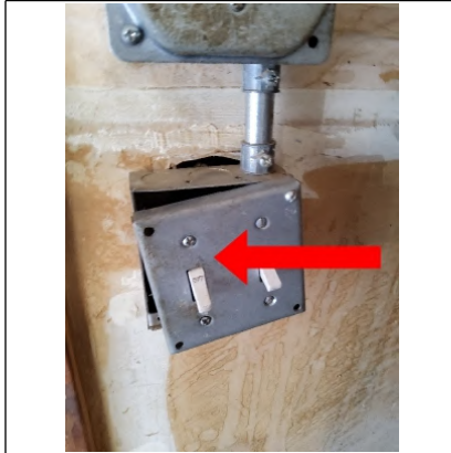
Loose switch cover
