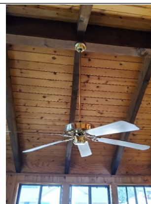
Ceiling fan is both loose and inoperable. Recommend having repaired by a Licensed Electrician.
