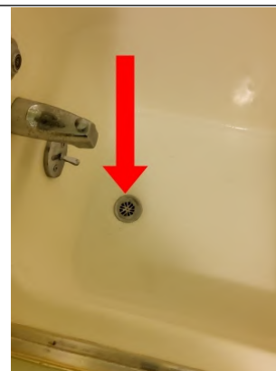
Drain is clogged
