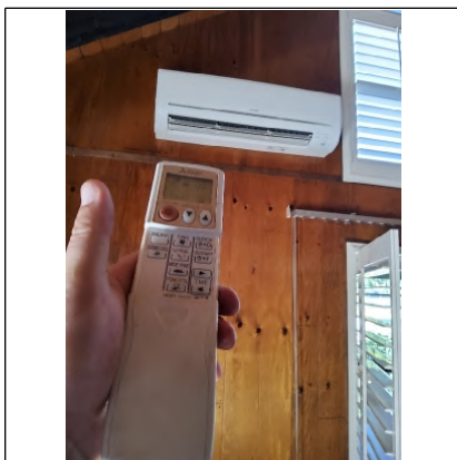
Remote Control shows proper operation when operating the air handler.
