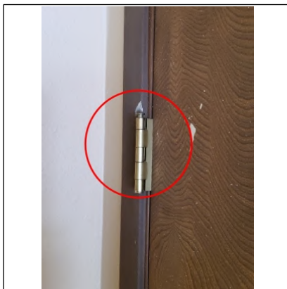
Recommend installing door stop.
