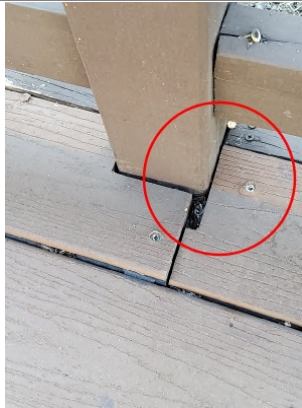
Poor quality work
