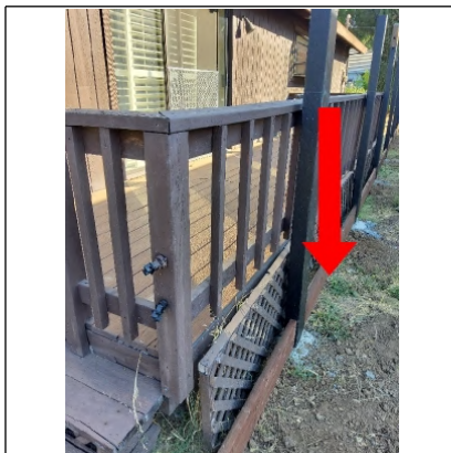
The deck is currently installed over the neighbors property line. Recommend contacting Hidden Valley Lake Association for proper deck set backs if an answer cannot be provided contact the Lake County Building Department.
