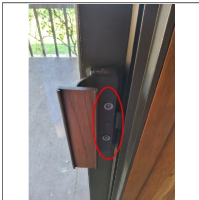
Recommend refastening loose door latch.
