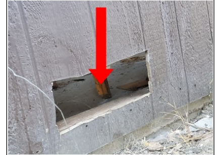
Rodent intrusion location. Recommend putting a new exterior vent cover on
