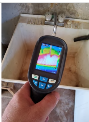
Thermal Imager shows hot water is present through faucet.
