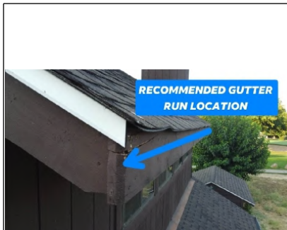
Recommend having a new gutter run installed on fascia member.
