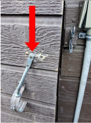
Missing screw on gate latch.
