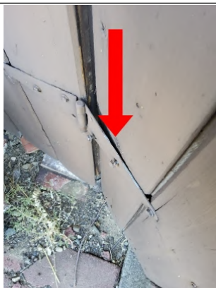
Loose gate hinge
