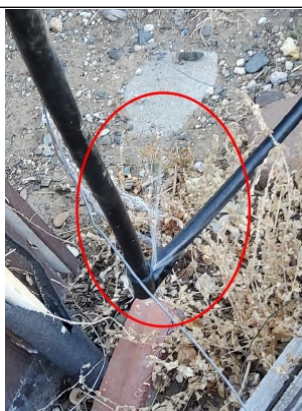
Damaged irrigation line
