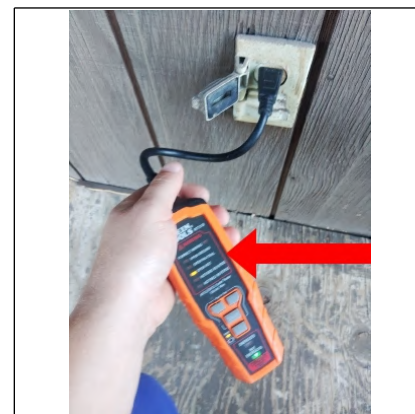
Electrical outlet is inoperable. Recommend having further evaluated and repaired by a Licensed Electrician.
