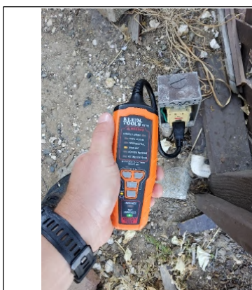
Electrical outlet is inoperable. Recommend having further evaluated and repaired by a Licensed Electrician.
