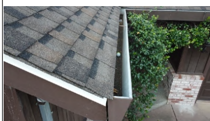
Gutter run has significant rust.
