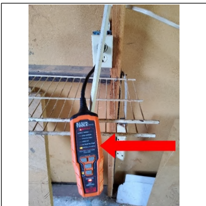
Electrical outlet has reverse polarity. Recommend having further evaluated and repaired by a Licensed Electrician.
