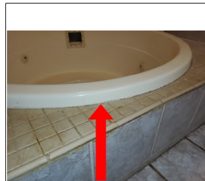
Recommend additional grout silicone be applied.
