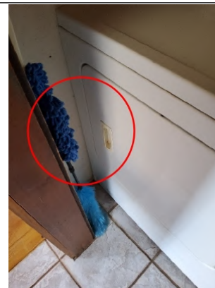
Dryer door will not open properly at its current location.
