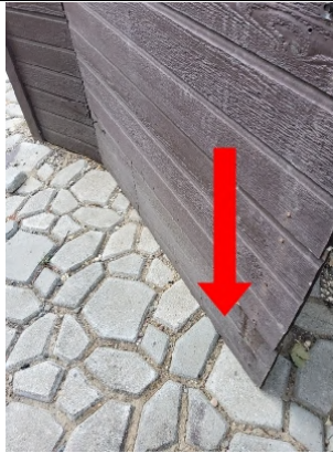
Recommend cutting down bottom portion of door flush to the bottom plate in order to properly swing door.
