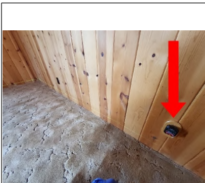
Electrical outlet is inoperable. Recommend having further evaluated and repaired by a Licensed Electrician.
