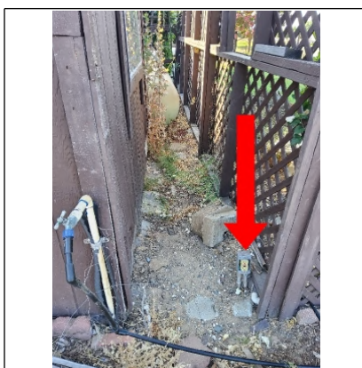
Missing exterior cover
