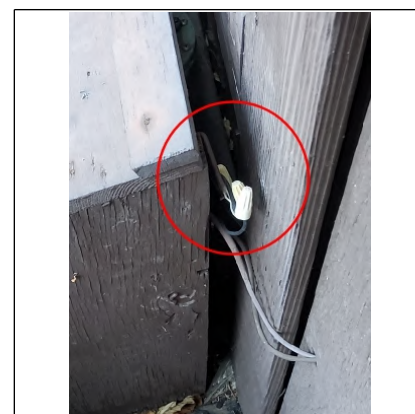
Exposed low voltage wires. Recommend having installed in a solid exterior junction box.
