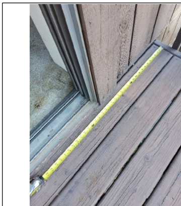
Joist layout is 32" on center which exceeds the minimum layout requires of 1-1/2" standard tread wood member layout.
