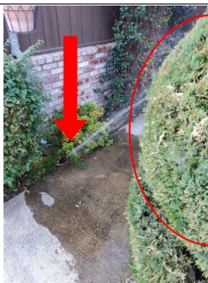
There is a rip in the irrigation line. However, this could be in purpose to water this bush.
