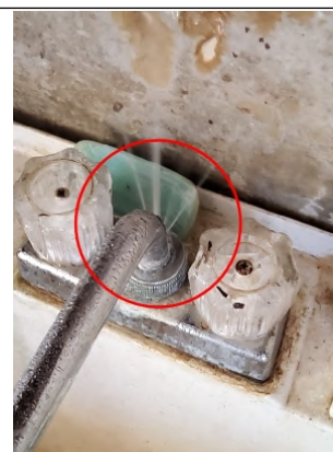
Recommend having damaged leaking faucet replaced by a Licensed Plumber.
