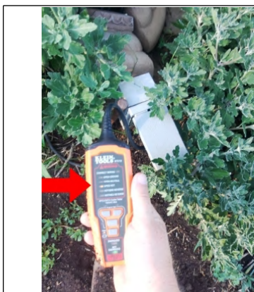
Electrical outlet is inoperable. Recommend having further evaluated and repaired by a Licensed Electrician.
