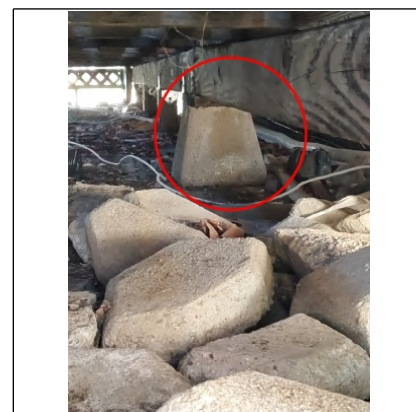
No footing appears to be present below pier blocks.
