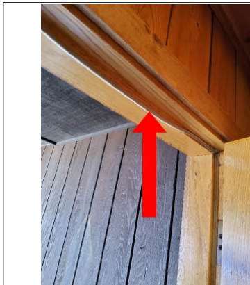
Recommend replacing weatherstripping.
