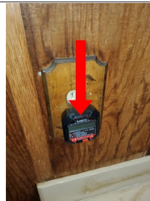
Electrical outlet is inoperable. Recommend having further evaluated and repaired by a Licensed Electrician.
