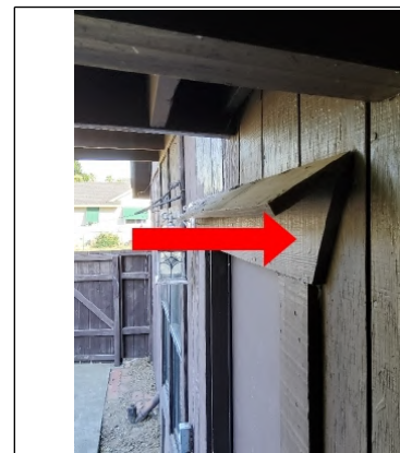
Recommend removing existing top trim member and install galvanized flashing above the existing casing trim.
