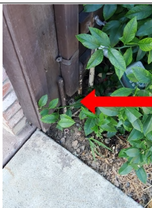
Missing downspout elbow
