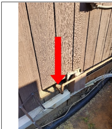
Recommend sealing off open vent location.
