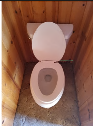
Toilet is loose at the base. Recommend having properly fastened to the floor from a Licensed Plumber.
