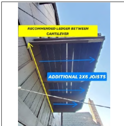
Recommend having a Licensed Contractor install ledger blocks between the cantilever joists as well as install 2x6 pressure treated joists to meet the minimum 2' on center joist layout for standard 1-1/2" wood tread members.
