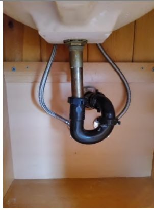
Sink drain line is not straight. Recommend having repaired by a Licensed Plumber.
