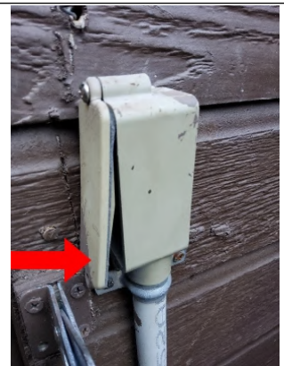
Missing screw on conduit cover.
