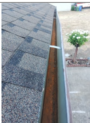
Gutter run has significant rust.
