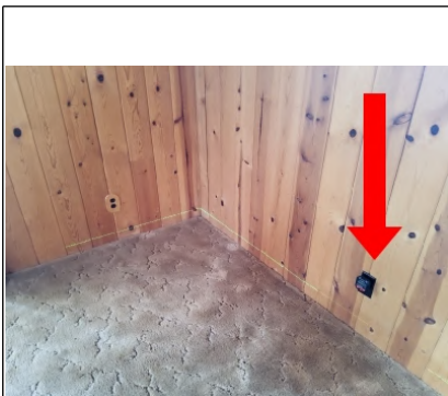
Electrical outlet is inoperable. Recommend having further evaluated and repaired by a Licensed Electrician.
