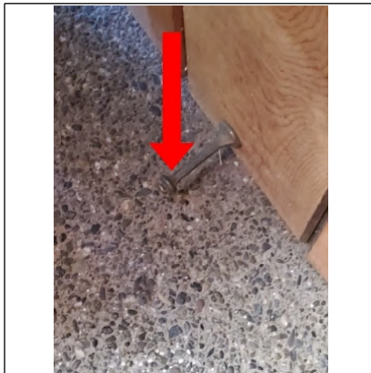
Missing rubber stopper on door stop.
