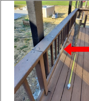
Railing is loose and should be properly refastened to the rim member of the deck but is also not required to have.
