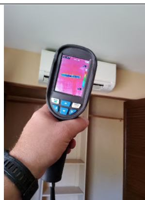
Thermal Reader shows air handler shows proper operation on "Cool" setting.
