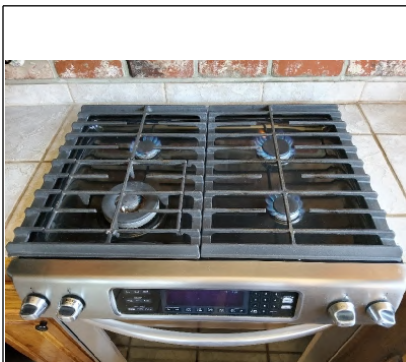
3 of the 4 burners show proper operation on the stove top.
