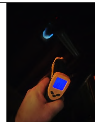
Thermal Reader shows 107.7 Degrees F at the roof vent location this shows there is proper ventilation and a satisfactory heat index.
