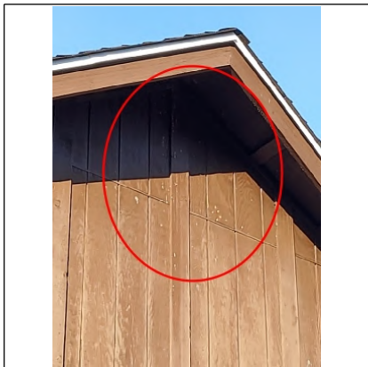
Woodpecker holes are evident on siding.
