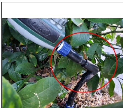
Leak on irrigation line
