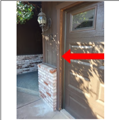
Recommend additional paint be applied on trim members.
