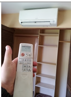
Remote Control shows proper operation when operating the air handler.
