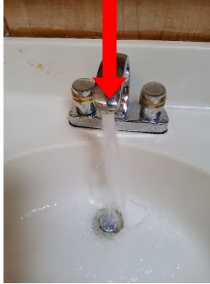
Recommend having aerator replace on faucet by a Licensed Plumber.
