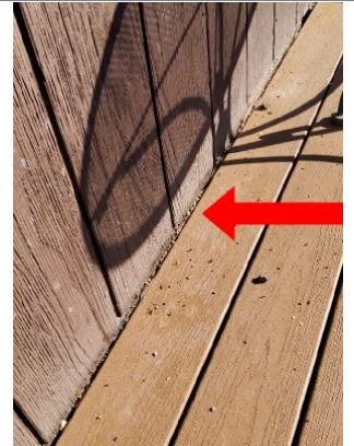
No flashing was installed on the ledger board prior to installing the Trex composite deck.
