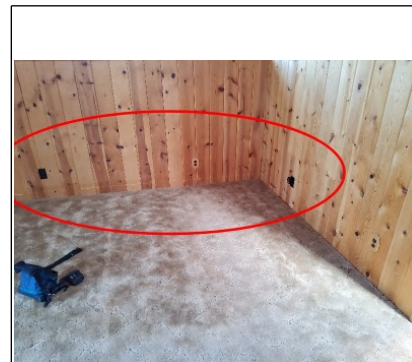
Noted electrical outlets are inoperable. Recommend having further evaluated and repaired by a Licensed Electrician.
